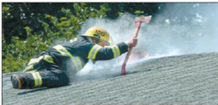
FIREFIGHTER of the West Berwick Hose Co. uses his ax to stop his fall as his left leg and arm break through the roof at 201 Maple Road in Berwick on Wednesday afternoon. Eveland suffered burns on both of his hands in the mishap during the attic fire. Press Enterprise/Ginny May
